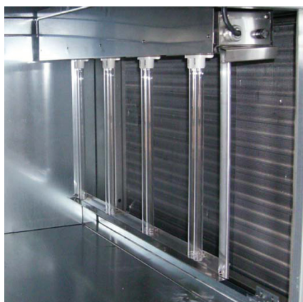
Figure 2: Typical in-duct UVGI installation with lamps mounted downstream of the cooling coil and drain pan.
